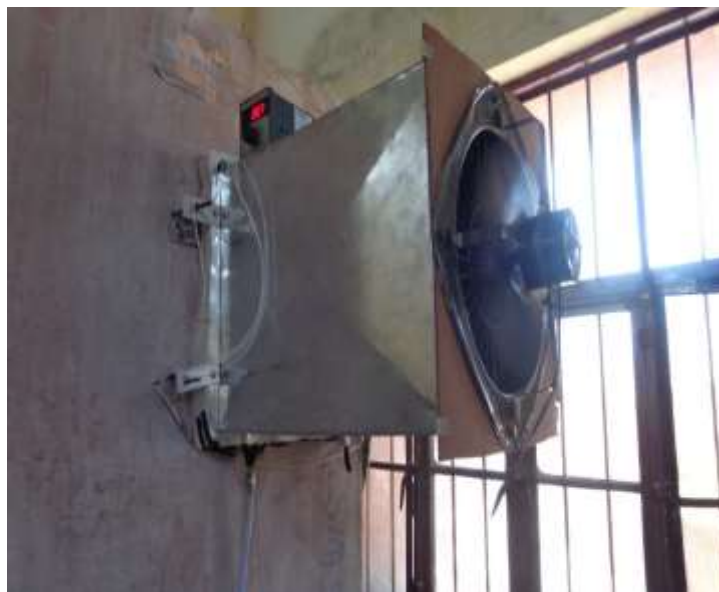
Fig.3: Air Conditioning Duct
